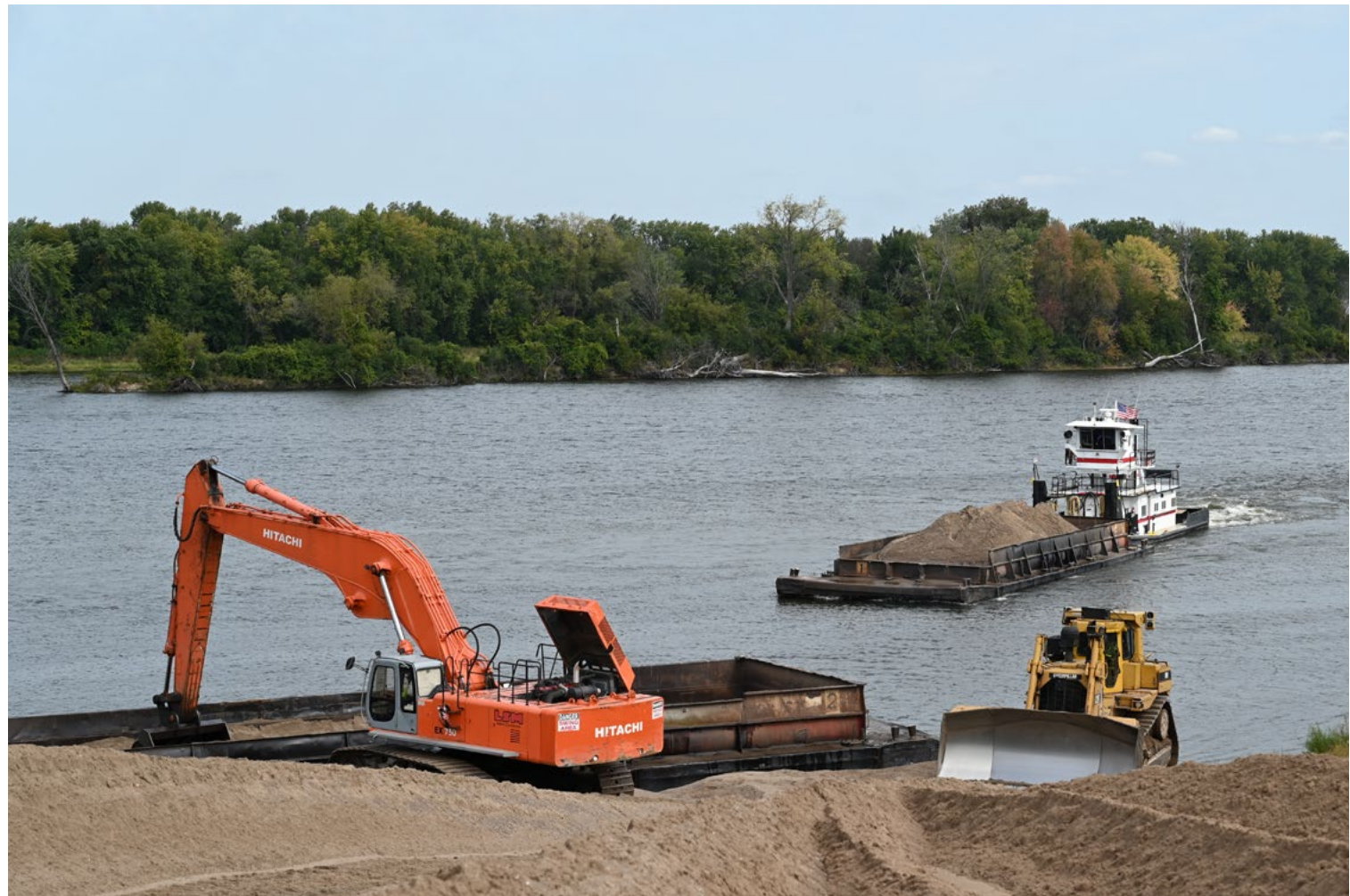
Dredging operations near La Crosse, Wisconsin, September 24, 2021. USACE photo by Patrick Moes
